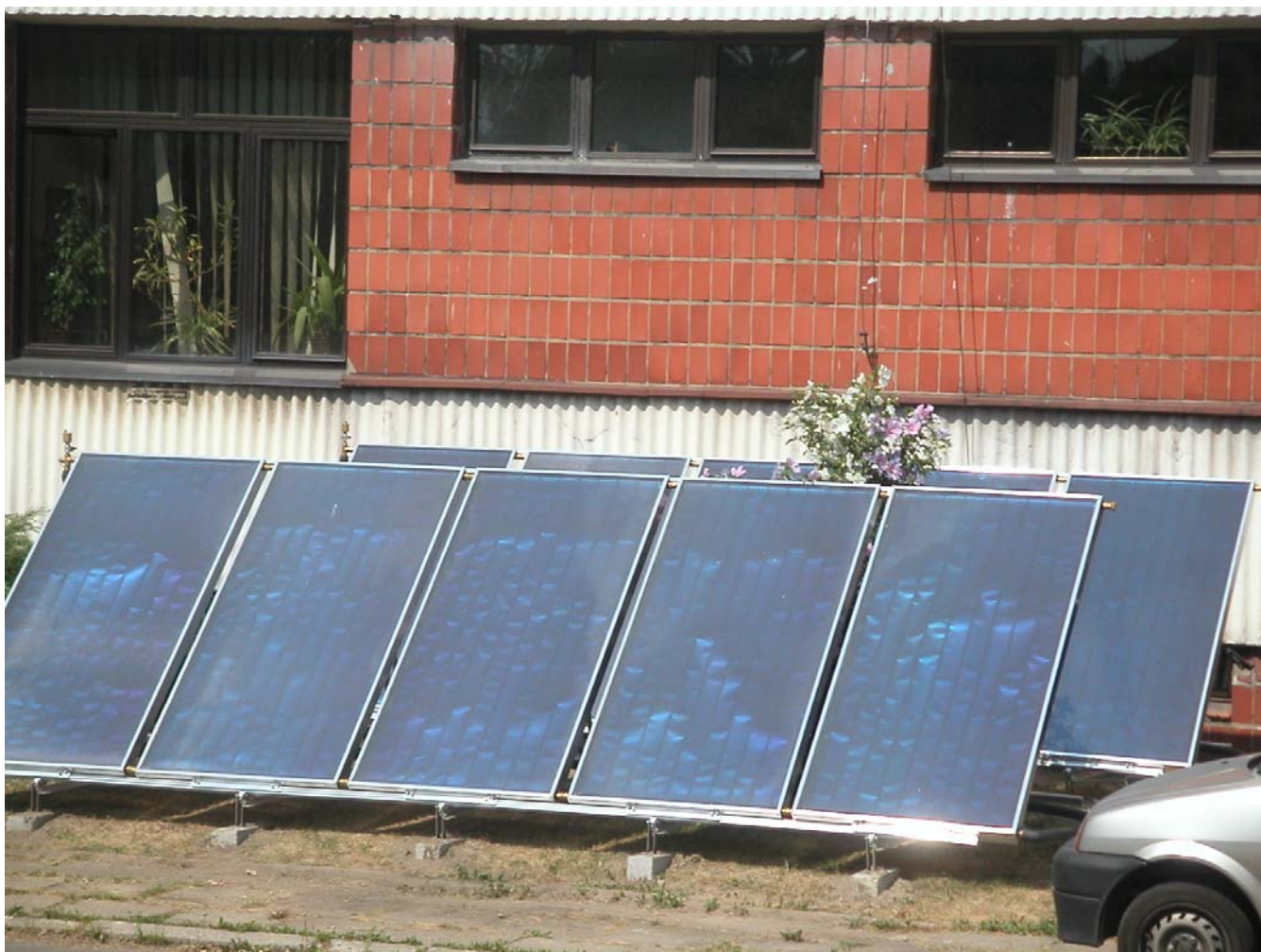
near view of the collectors
